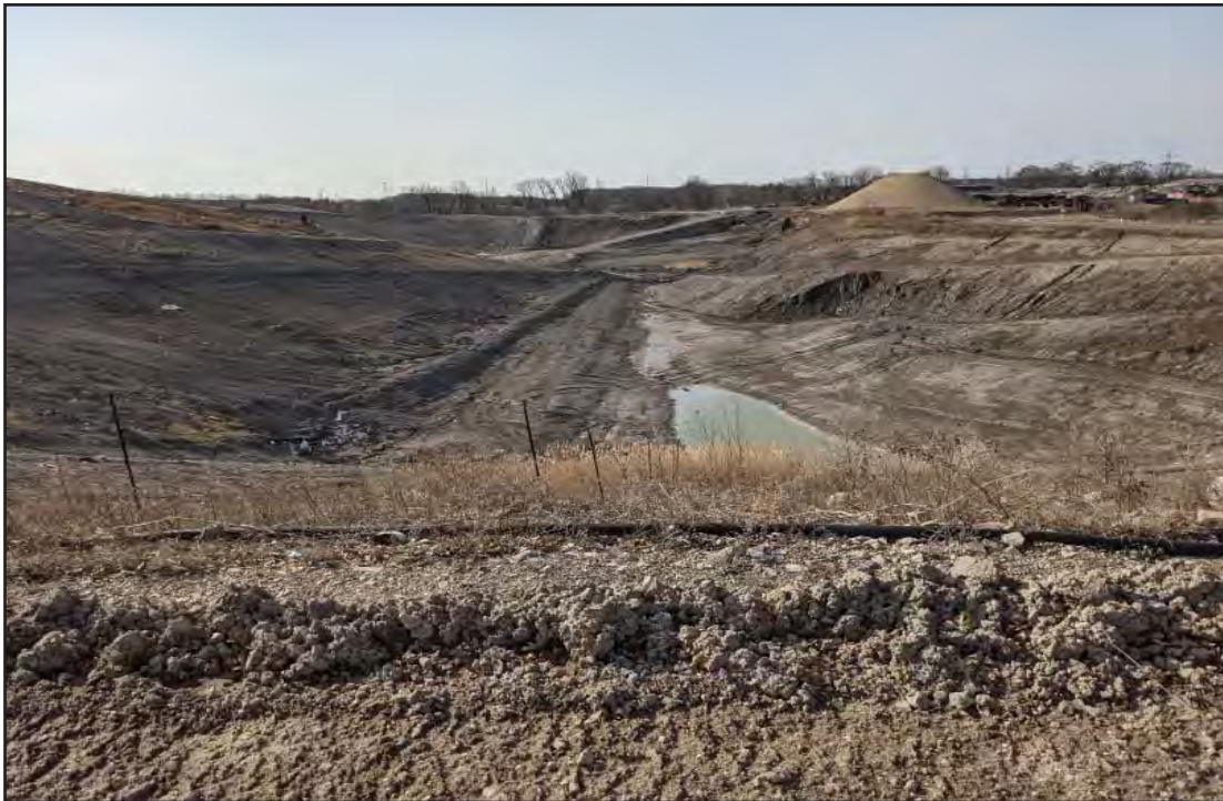
Temp sed basin and West slope of Phase 7 viewed from the North
