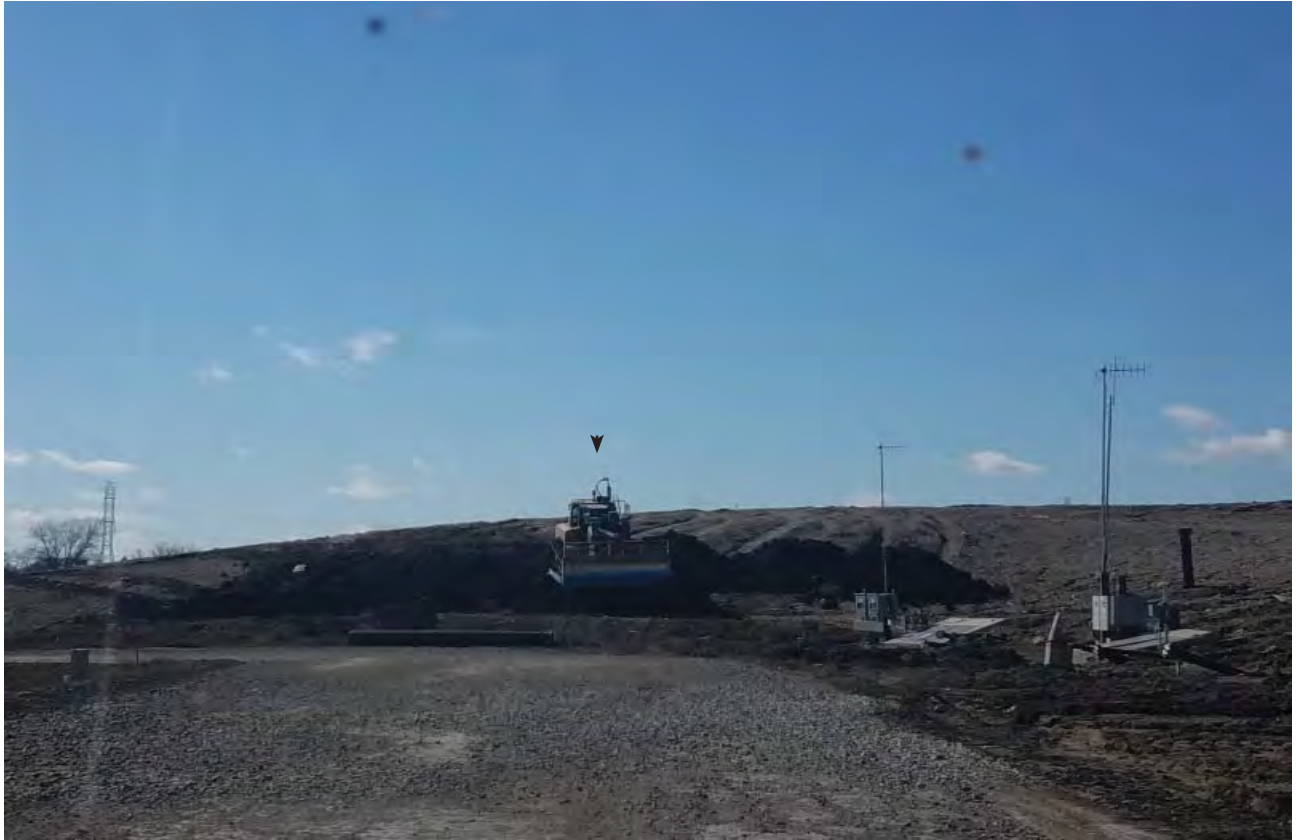
South slope of Phase 7. Berm being placed to control and slow runoff from upper slopes.
