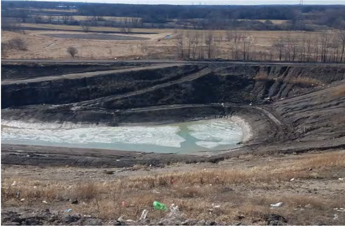
Temp sed basin, pump is placed and the basin is well emptied
