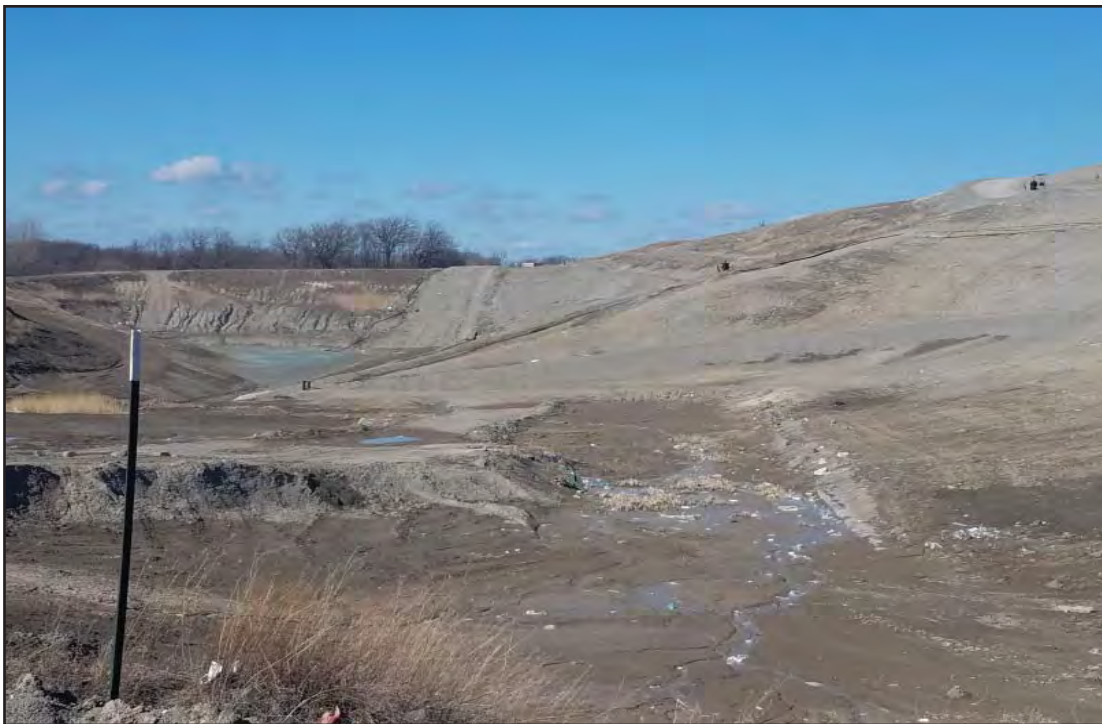
West slopes of Phase 7, temp sed basin in the far end of picture
