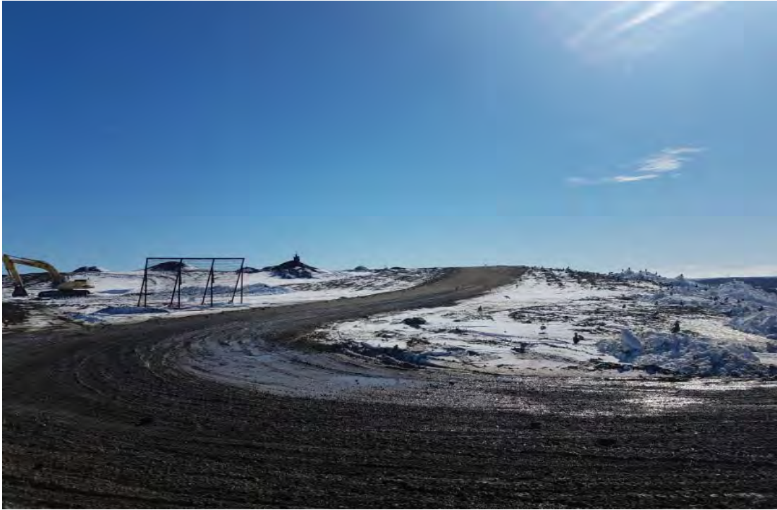
Phase 7, berm about top of Phase to allow waste placement in inclement weather
